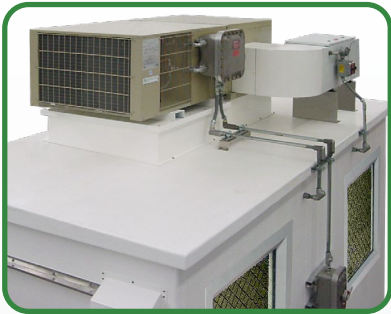
A Bebco Model RMP supplies a Bebco Model PAC Unit to protect this Refinery Gate Security Center
