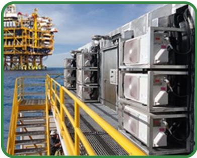
An Offshore Drilling Rig Crew Quarters Balcony features 27 Bebco Model SAC Split System Condenser Units
